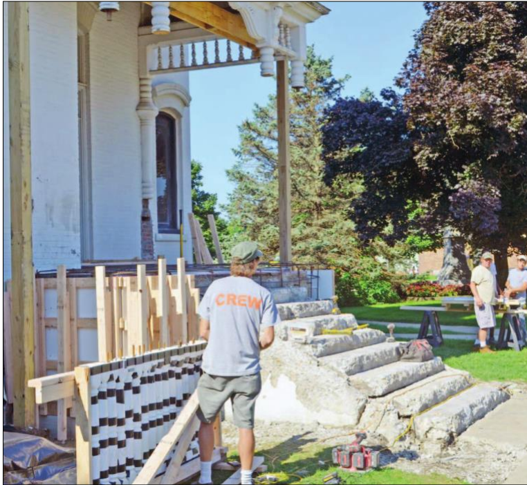
The original Coldwater Library steps and porch were recently remove and replaced with modern concrete. Dynamic Hardscapes and Construction moulded its own concrete balusters in the black and white tubes to replace the ones that were crumbling. DON REID PHOTO
