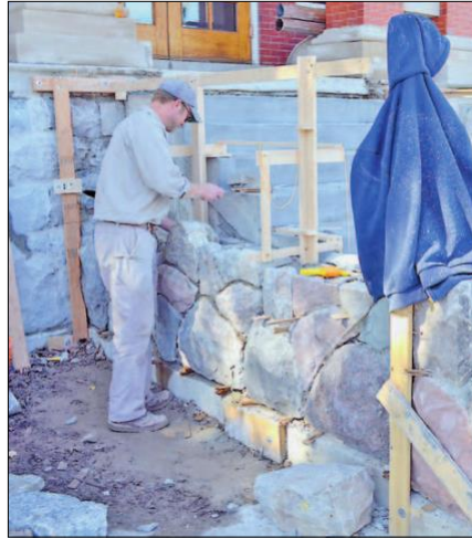
Stone mason Chris Devries of Grand River Builders replaces stone on the Quincy Library steps during his months of work. DON REID PHOTO
