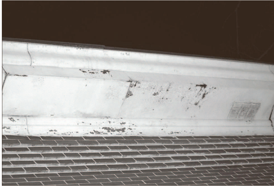
The rusted eaves and gutter on the Quincy Library. DON REID PHOTO
