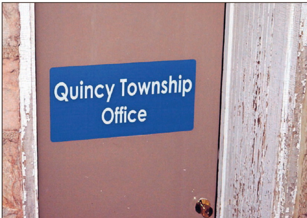
The rotted wood door frame at the Quincy Library. DON REID PHOTO
